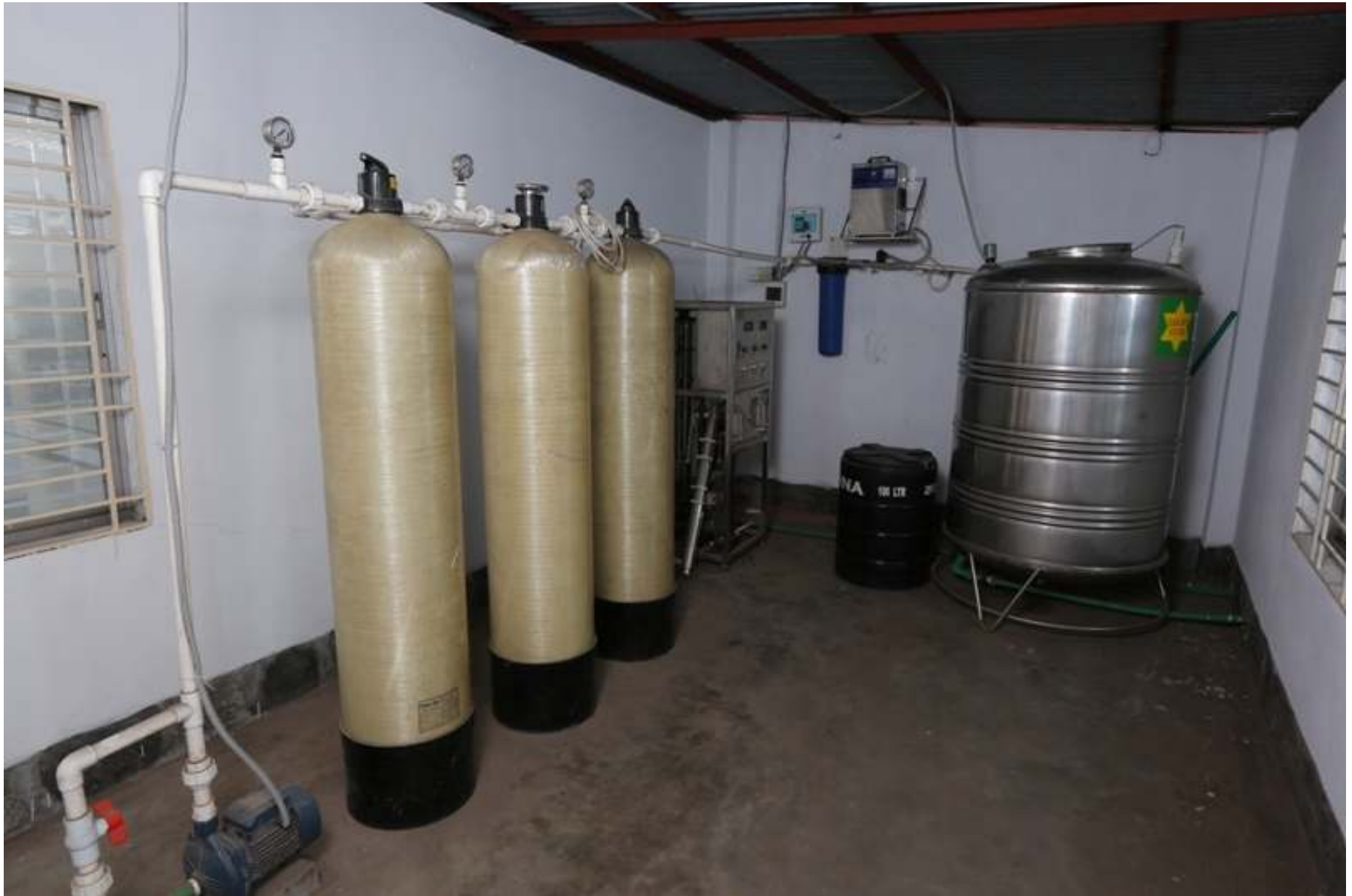
Drinking water purification system
