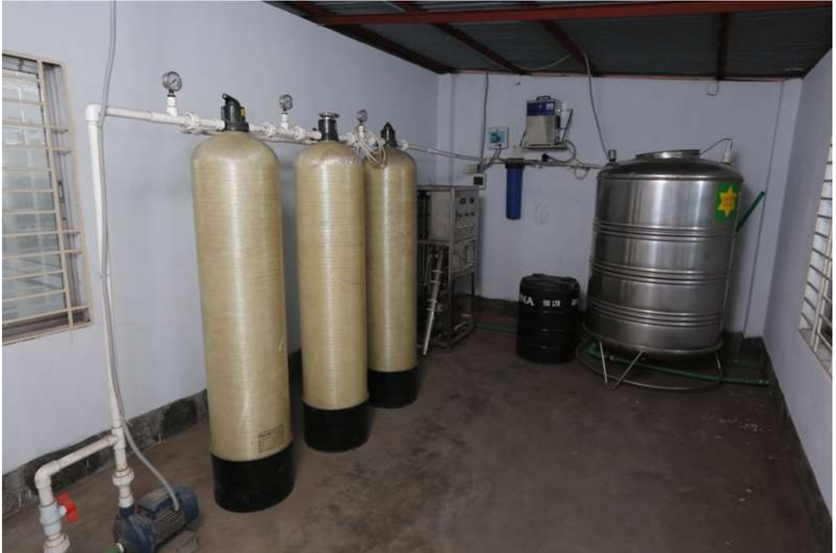
Drinking water purification system
